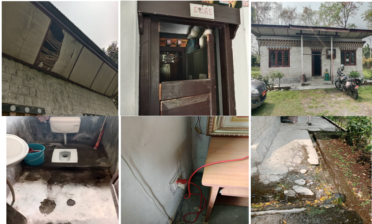
Figure 1 Pictures showing dilapidated Sarpang Range Office.
