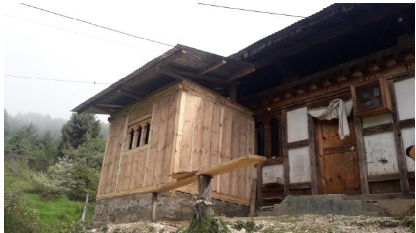
Fig:1 Sample of kitchen to be attached on staff quarter in Head office, Ura.
