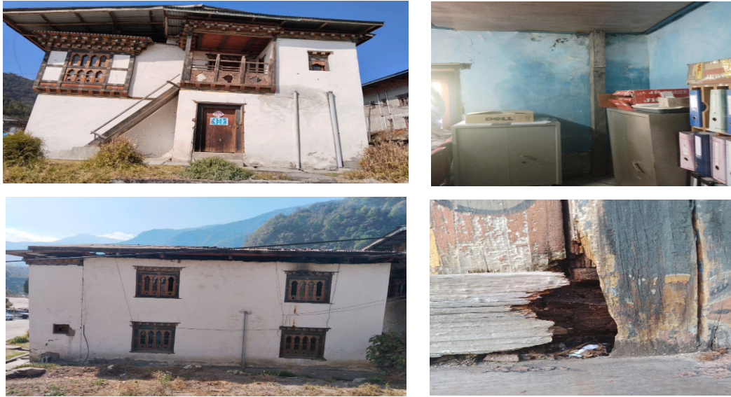
Figure 5. Condition of Range Office, Trashiyangtse
