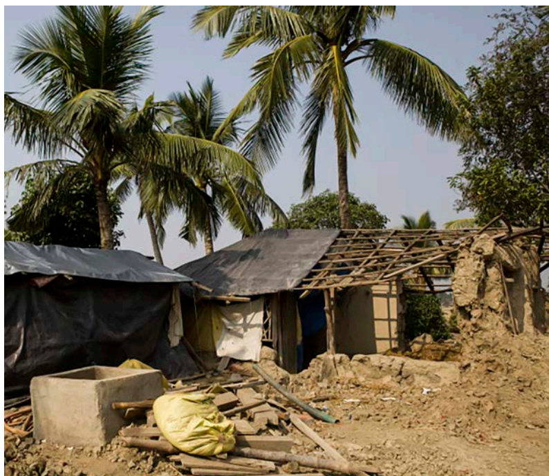
A house damaged by the most recent cyclone, Mousuni Island, Sundarbans, India
