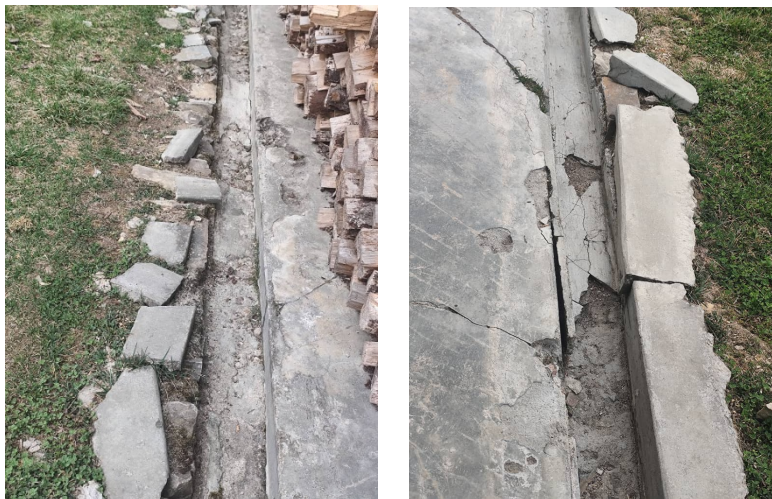
Figure 2: Current condition of the Drain
